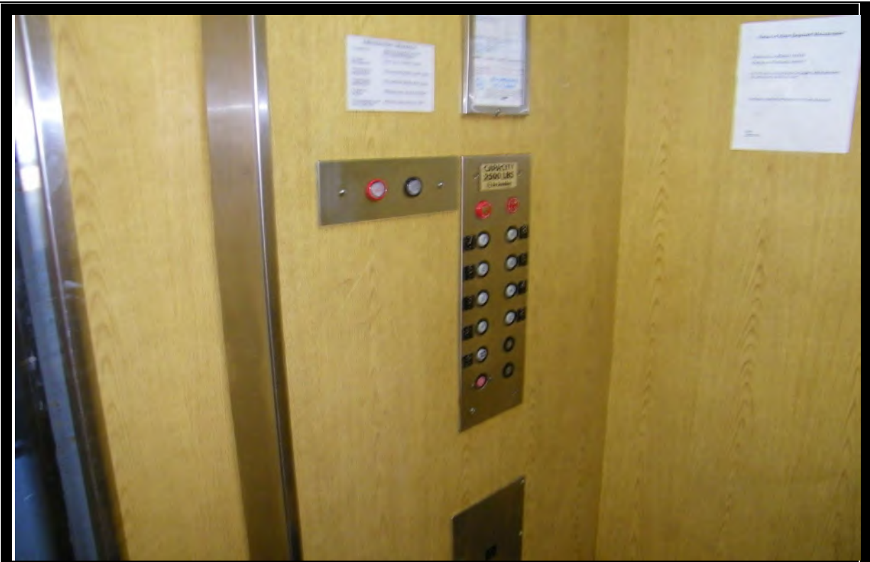
VIEW OF TYPICAL BUILDING MECHANICAL EQUIPMENT
