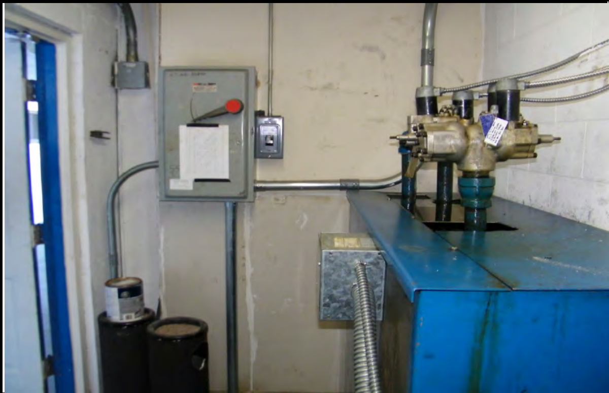
VIEW OF TYPICAL BUILDING MECHANICAL EQUIPMENT
