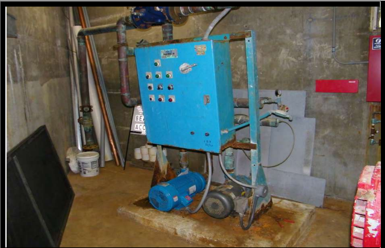
VIEW OF TYPICAL BUILDING MECHANICAL EQUIPMENT
