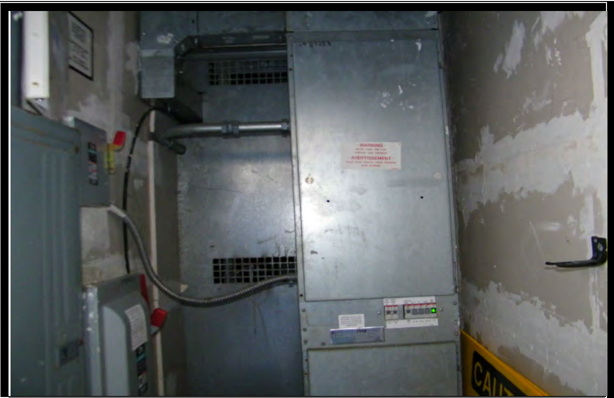
VIEW OF TYPICAL BUILDING MECHANICAL EQUIPMENT
