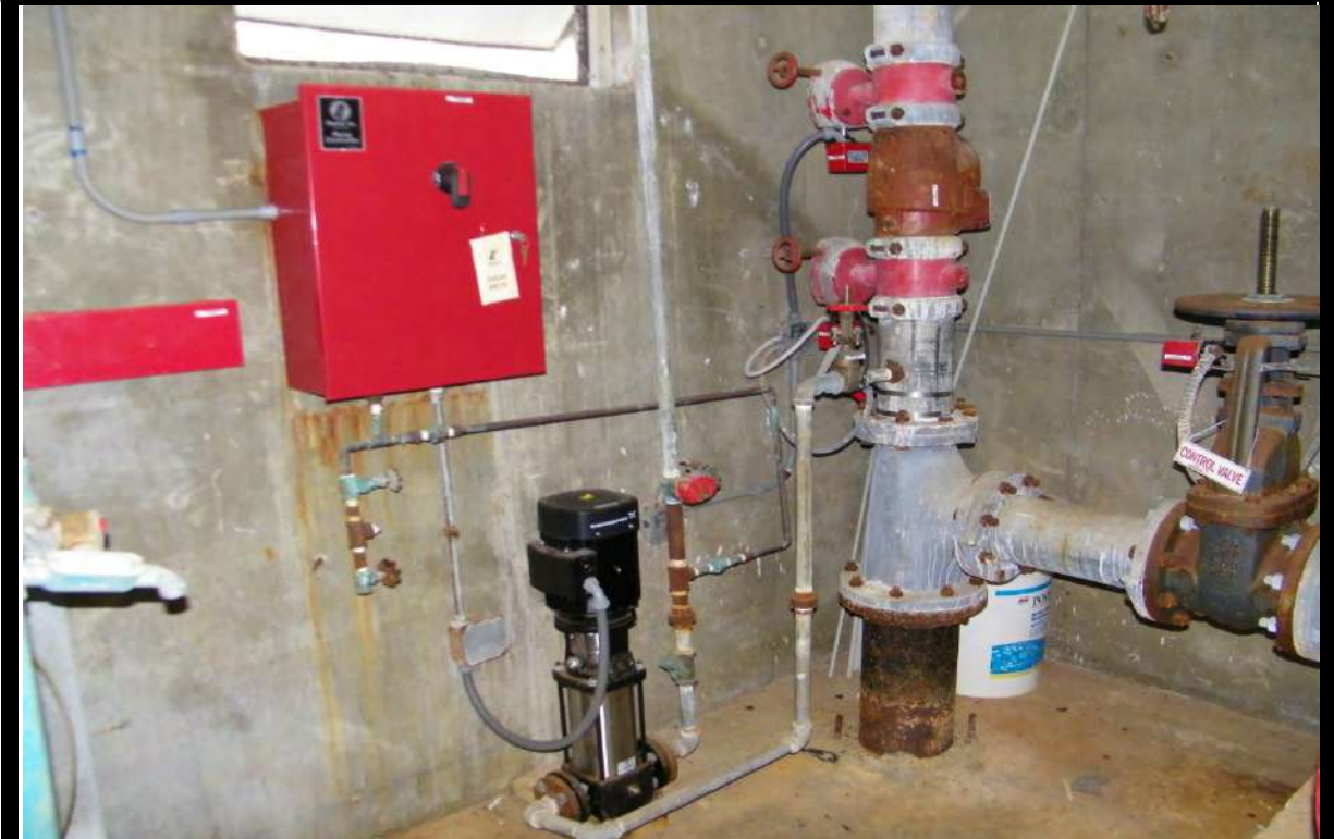
VIEW OF TYPICAL BUILDING MECHANICAL EQUIPMENT
