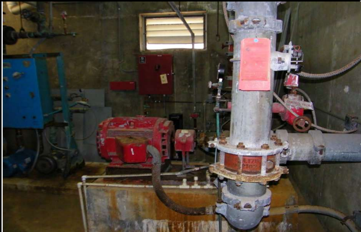
VIEW OF TYPICAL BUILDING MECHANICAL EQUIPMENT
